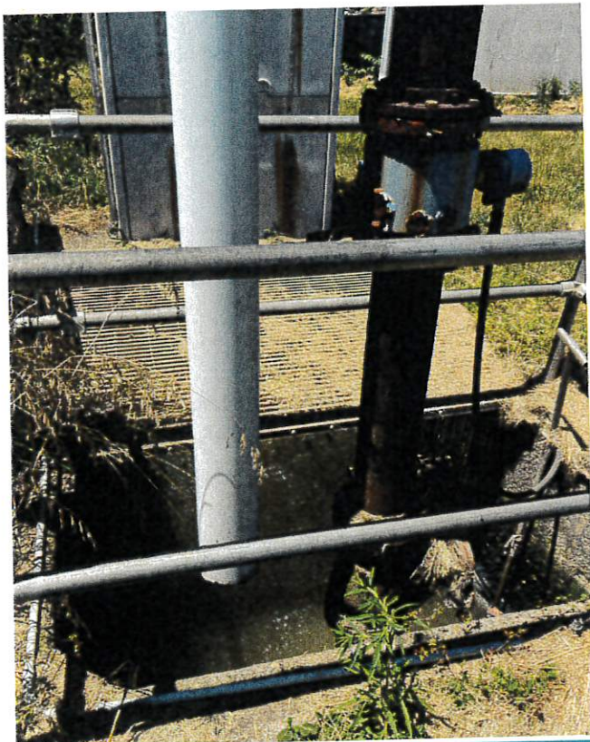
Influent junction box at headworks with Junaluska Sanitary District force main connection
