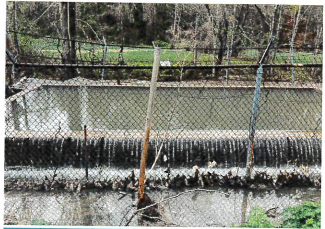
Hurricane Helene completely flooded the Little Champion wastewater junction box.
